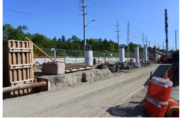
MAY: The foundation work for the North-South Pedestrian-Cyclist Crossing at Premium Way.
