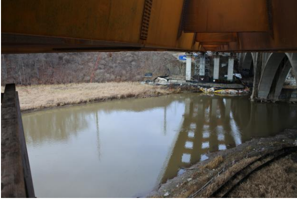
JANUARY: The girders are installed for the New QEW Credit River Bridge – looking at the underside.
