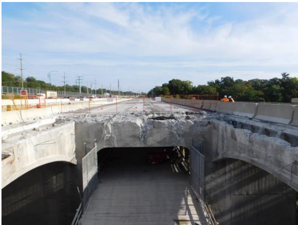
SEPTEMBER: The start of the removal of the existing QEW bridge deck.
