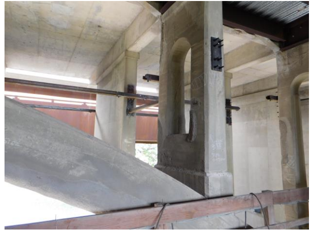
SEPTEMBER: Existing QEW bridge substructure bracing, the first step in the bridge rehabilitation.
